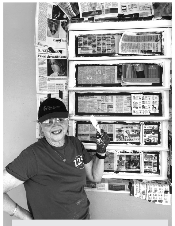
Nancy Hatcher on the job! Painting louvres after masking with newspaper, as part of hurricane damage repair in Maunabo, Puerto Rico. Photo courtesy of Nancy Hatcher
