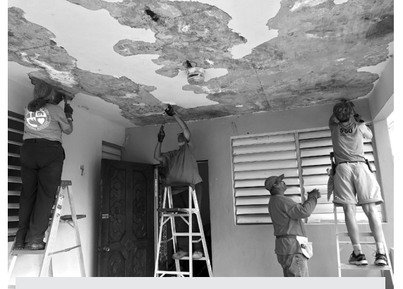
Volunteers work to repair hurricane damage in Maunabo, Puerto Rico. Photo courtesy of Nancy Hatcher
