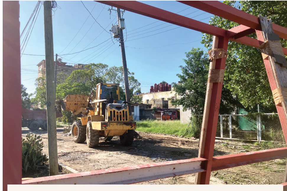
The day after the hurricane, working crews started clearing debris and restoring posts and lines. Photo by Leni Villagomez Reeves
